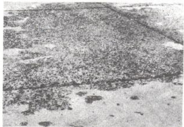
Scaling concrete surface.
