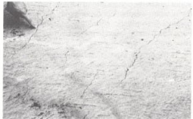
Plastic Shrinkage Cracks
